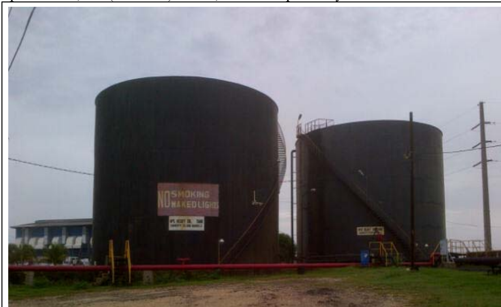
Photo 7 – HFO Tank #1 and 2
