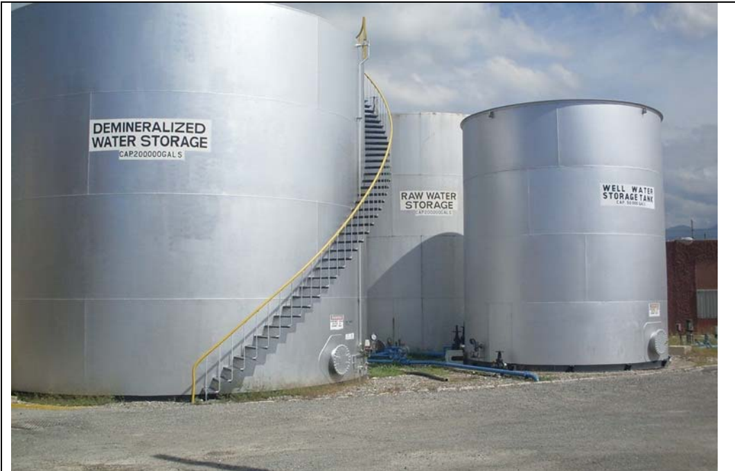
Photo 6 – Hunts Bay B6 – Demin Water Tanks
