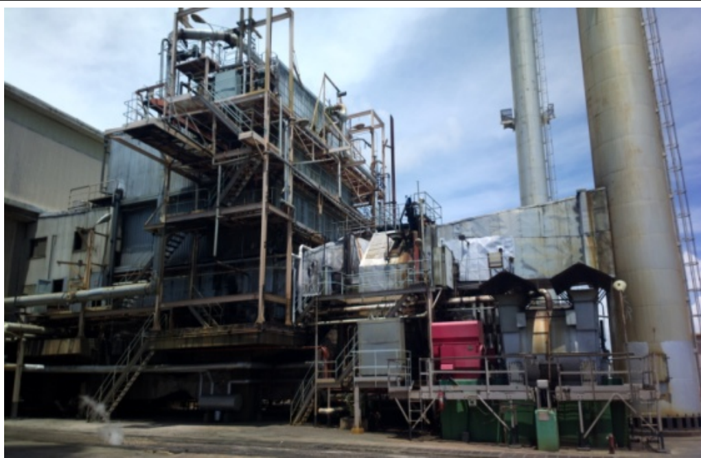
Photo 6 - A section of a boiler
