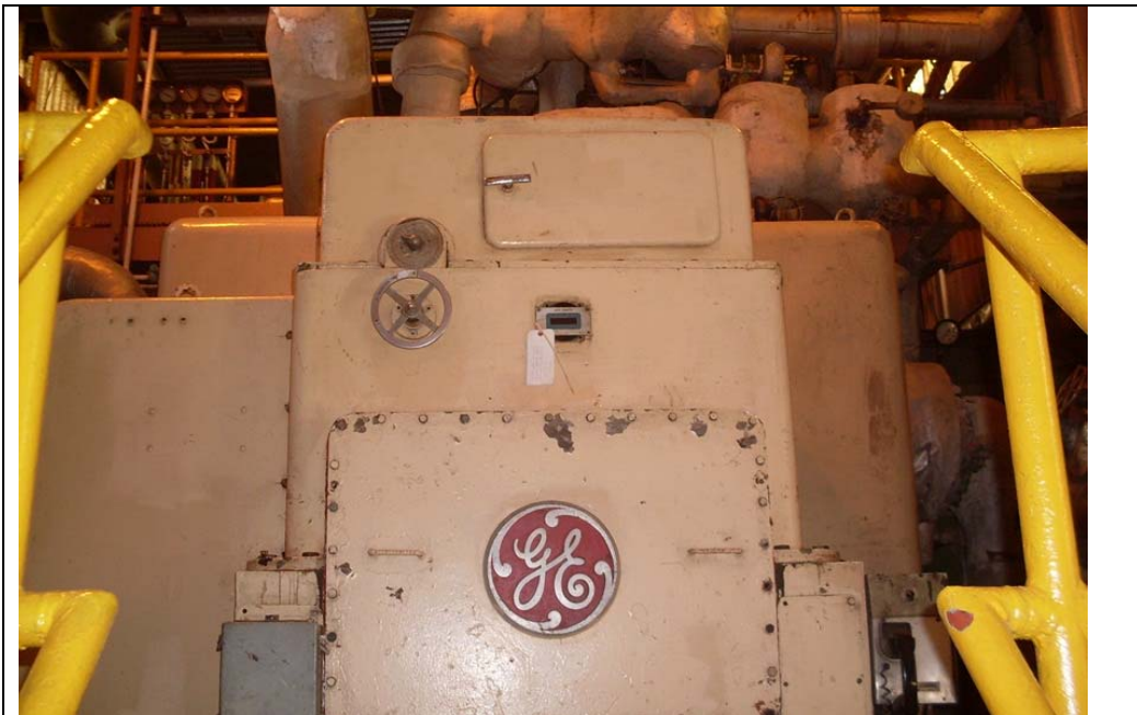
Photo 7 – Hunts Bay Unit B6 – Turbine front Standard Control Compartment
