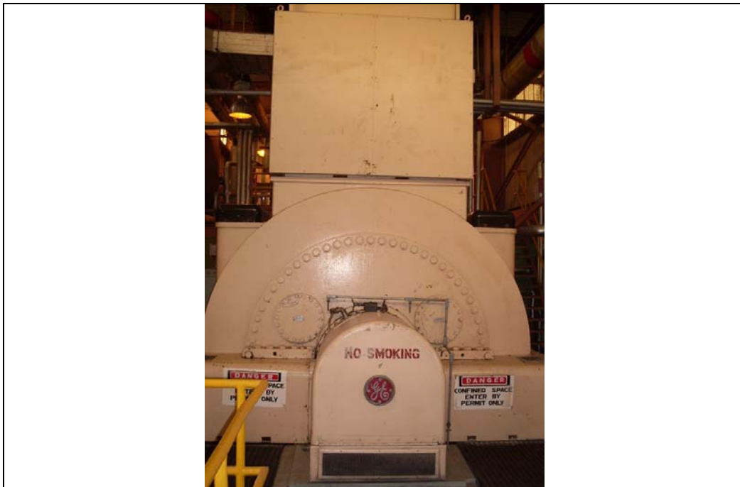
Photo 7 – Hunts Bay B6 Generator Casing
