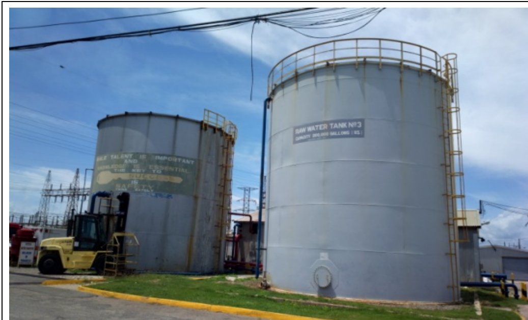
Photo 9 - Raw water tanks #1 and 3
