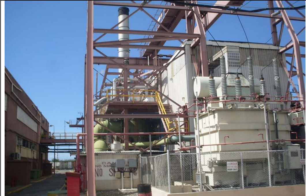
Photo 6 – Hunts Bay – Unit B6 transformer
