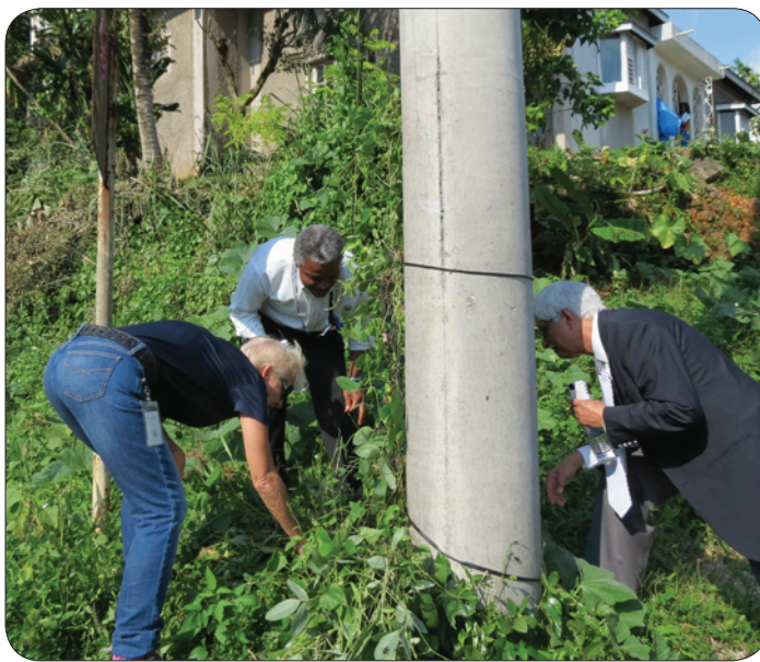
OUR Director General Zia Mian (right), JPS President and CEO Kelly Tomblin (left) and Head of Government and Regulatory Affairs at the JPS Sam Davis (centre) unearth what appears to be an illegal connection during a tour of Stony Hill St. Andrew to observe electricity restoration efforts following the passage of Hurricane Sandy.
