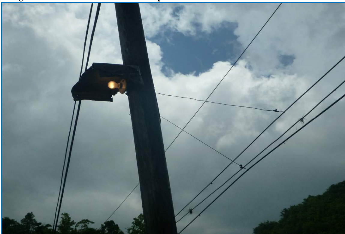
Figure 10.75: Makeshift Street Lamp On JPS Pole
