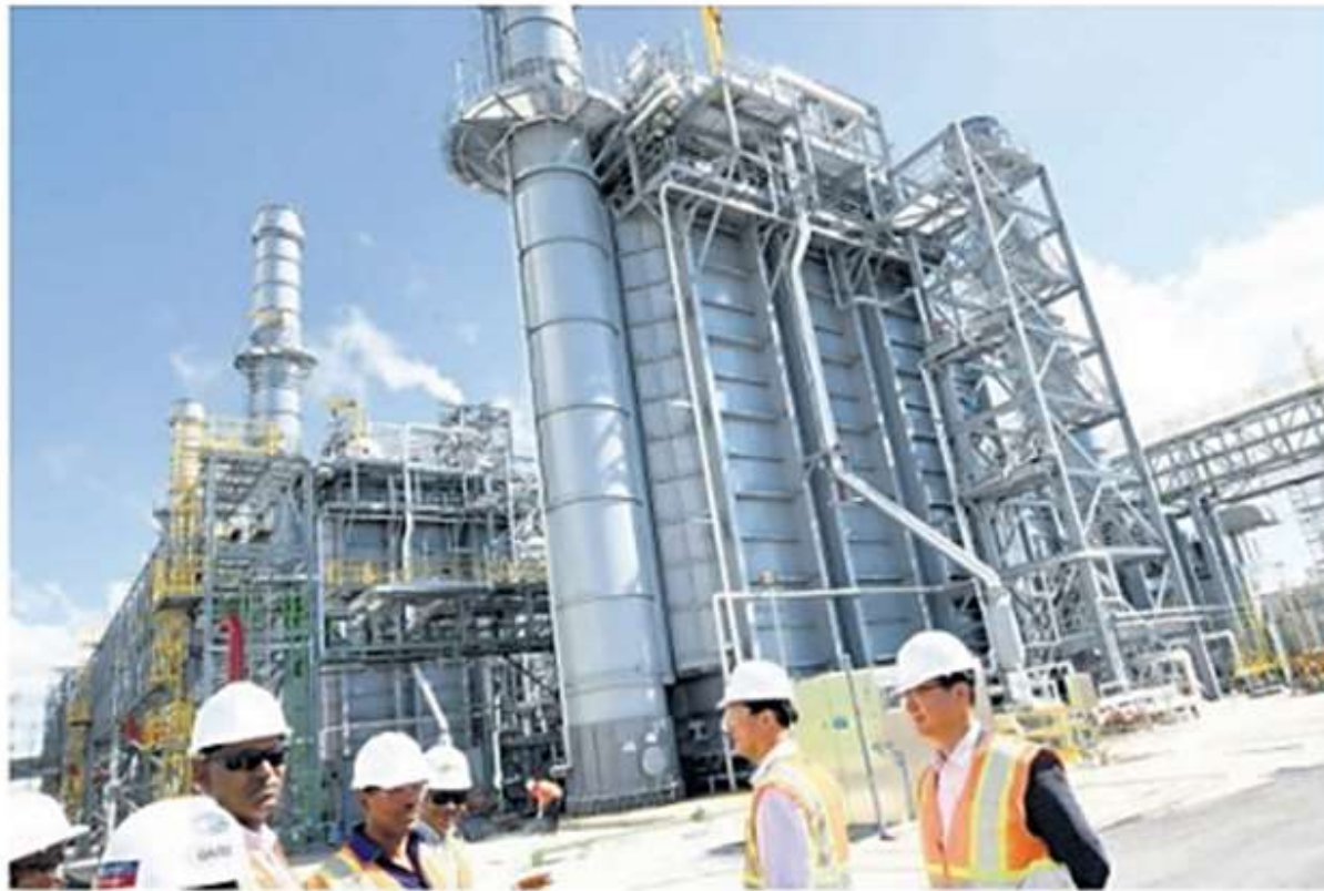
In forefront are members of the management team of the Jamaica Public Service Company during a media tour of the 190-megawatt power plant at Old Harbour Bay, St Catherine, on January 9, 2020.
