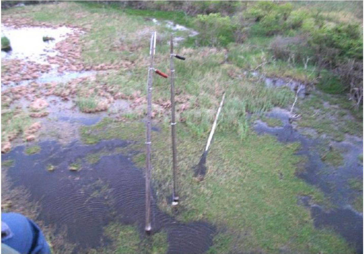
Picture showing fallen pole on structure # 18 on JPS Tredegar to Duhaney 138 kV transmission line
